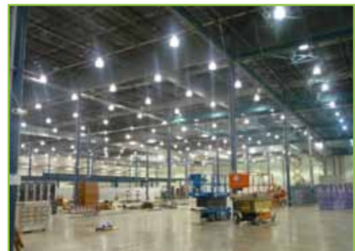
After Metrolight 250w SmartHID™ electronic ballasts - matching light levels!
